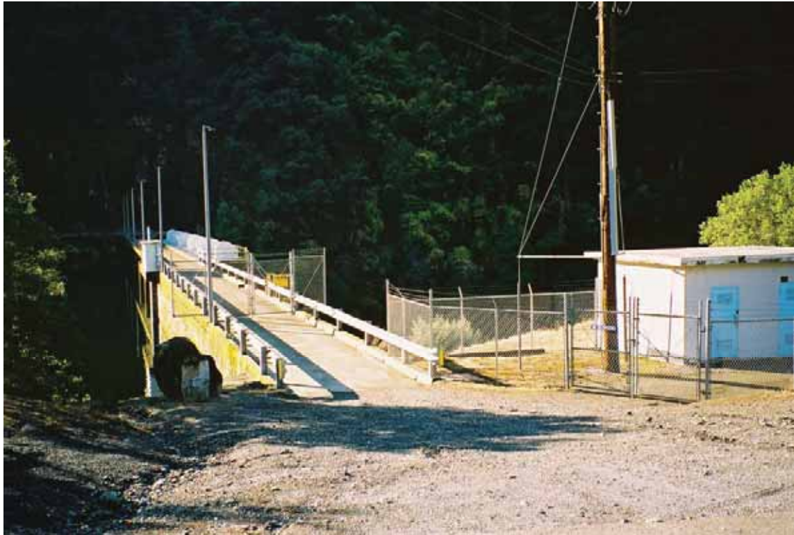
Photo M-3. View of safety railing across Ralston Afterbay Dam and perimeter fencing around the Ralston Afterbay Dam Generator Building. Also note locked fence and gate to prohibit access to dam.
