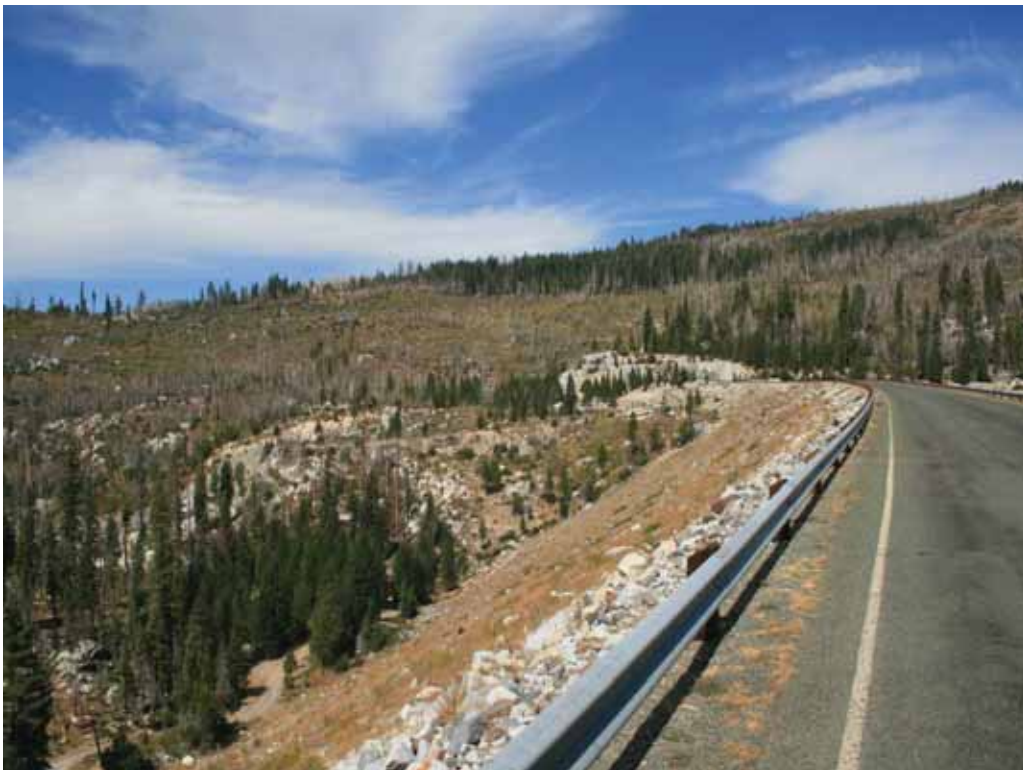
Photo J-4. View of guard rail along top of French Meadows Dam.
