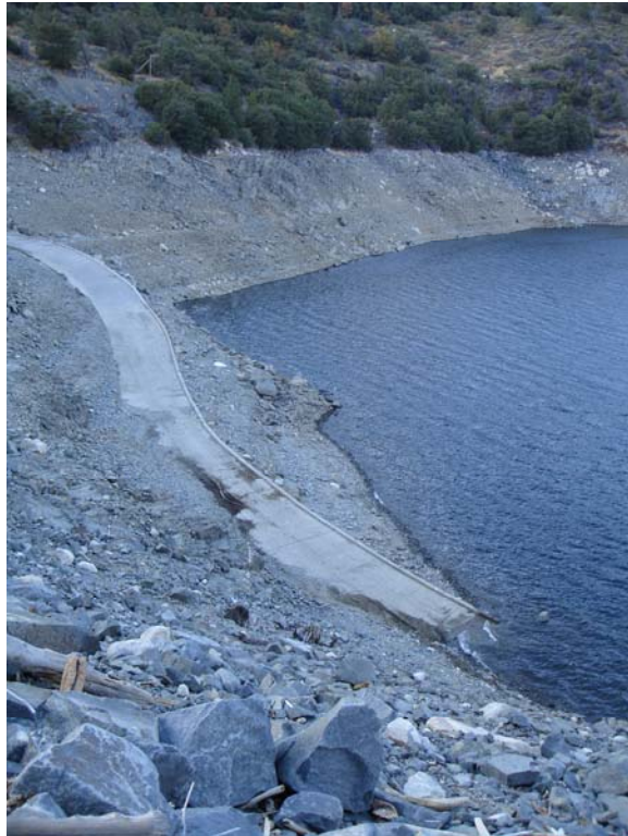
Photo B-5. View of Hell Hole Boat Ramp as viewed from edge of Hell Hole Boat Ramp Parking Area (October 5, 2009, WSE = 4,547 ft)
