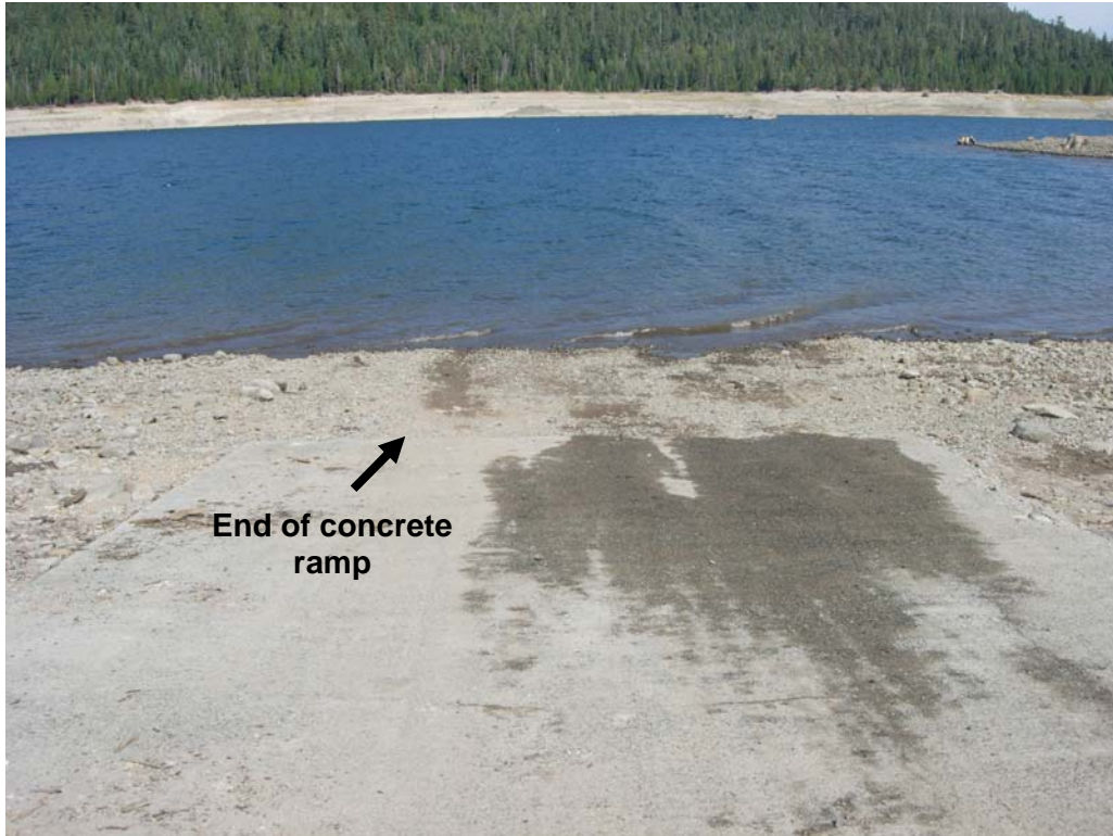
Photo G-5. French Meadows Boat Ramp on September 24, 2008 (WSE = 5,198 ft). The concrete ramp terminates at 5,200 feet.
